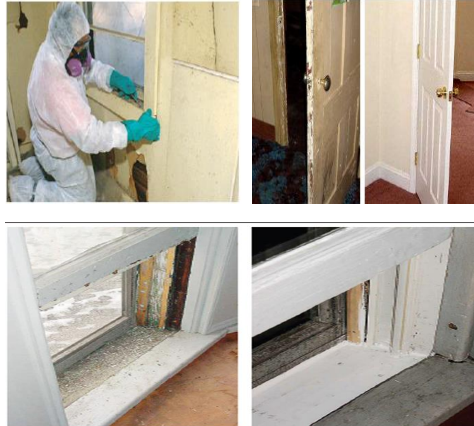
FIGURE 11.3 Window before and after friction treatment.
